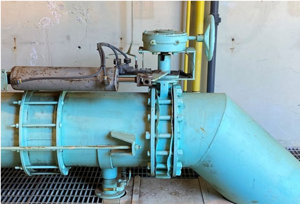
Filter Rate Control Valve Assembly – Filter #4, SGTP
