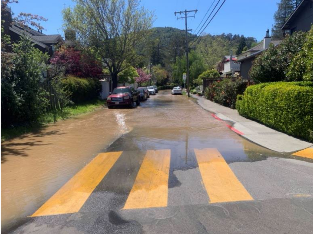
Water Main Break
