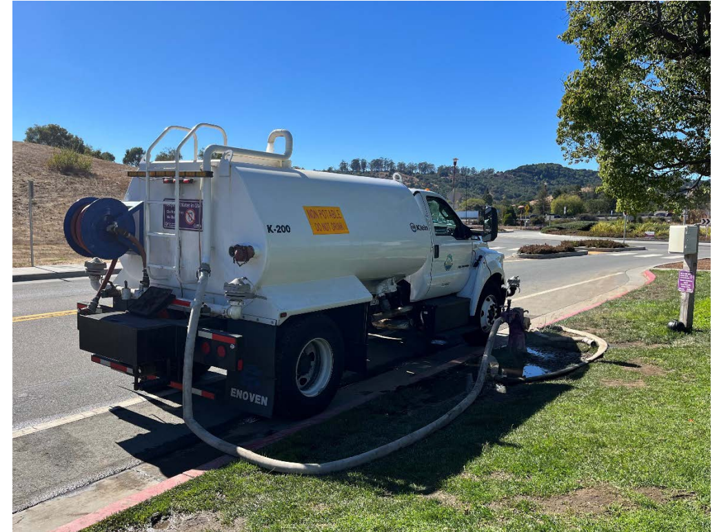
Sanitary agency filling up with recycled water for sewer cleaning near Civic Center Drive
