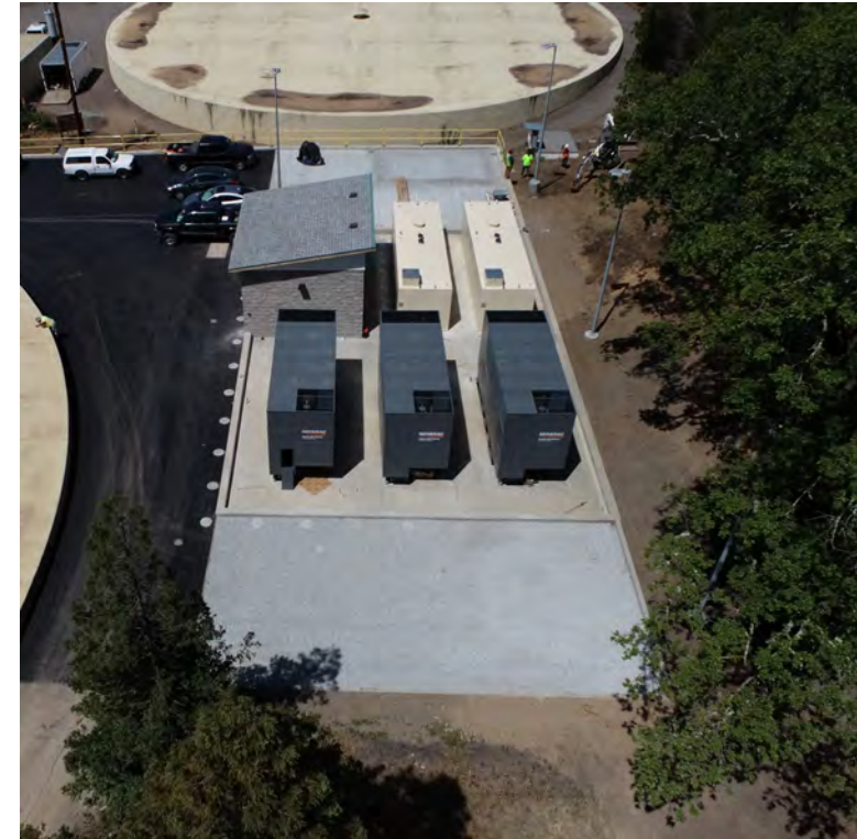
San Geronimo Permanent Generators
