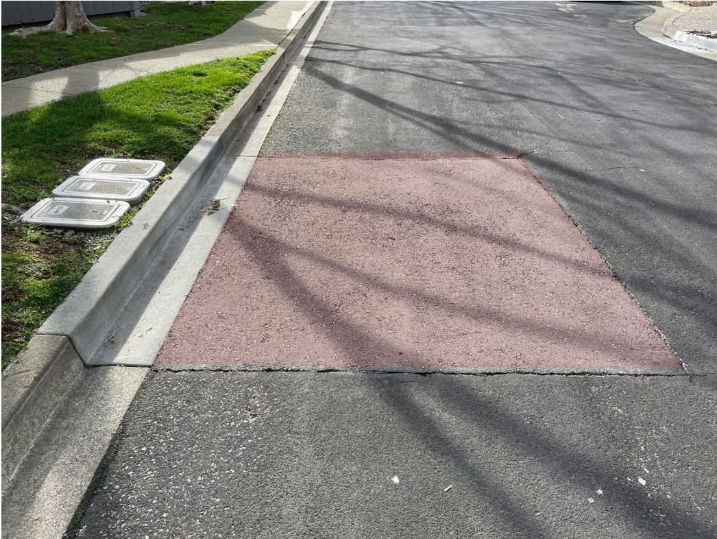
PRE-2018 MARIN COUNTY UCS PAVING PATCH
